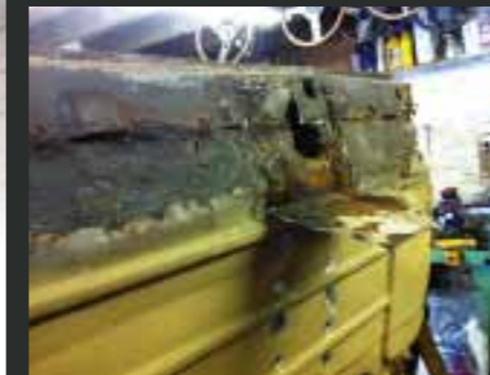
Bodged sill sections and outer floors had to be replaced. You can see marks where the floor crossmember has been removed and the front end is also absent here.
